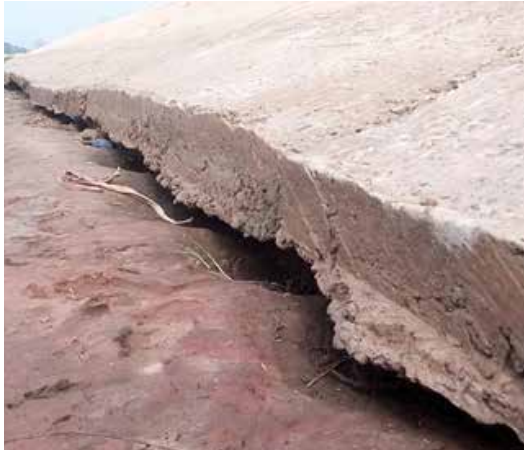
Picture 7: Seepage into the Ohawu Dam wall base resulting in project halt
